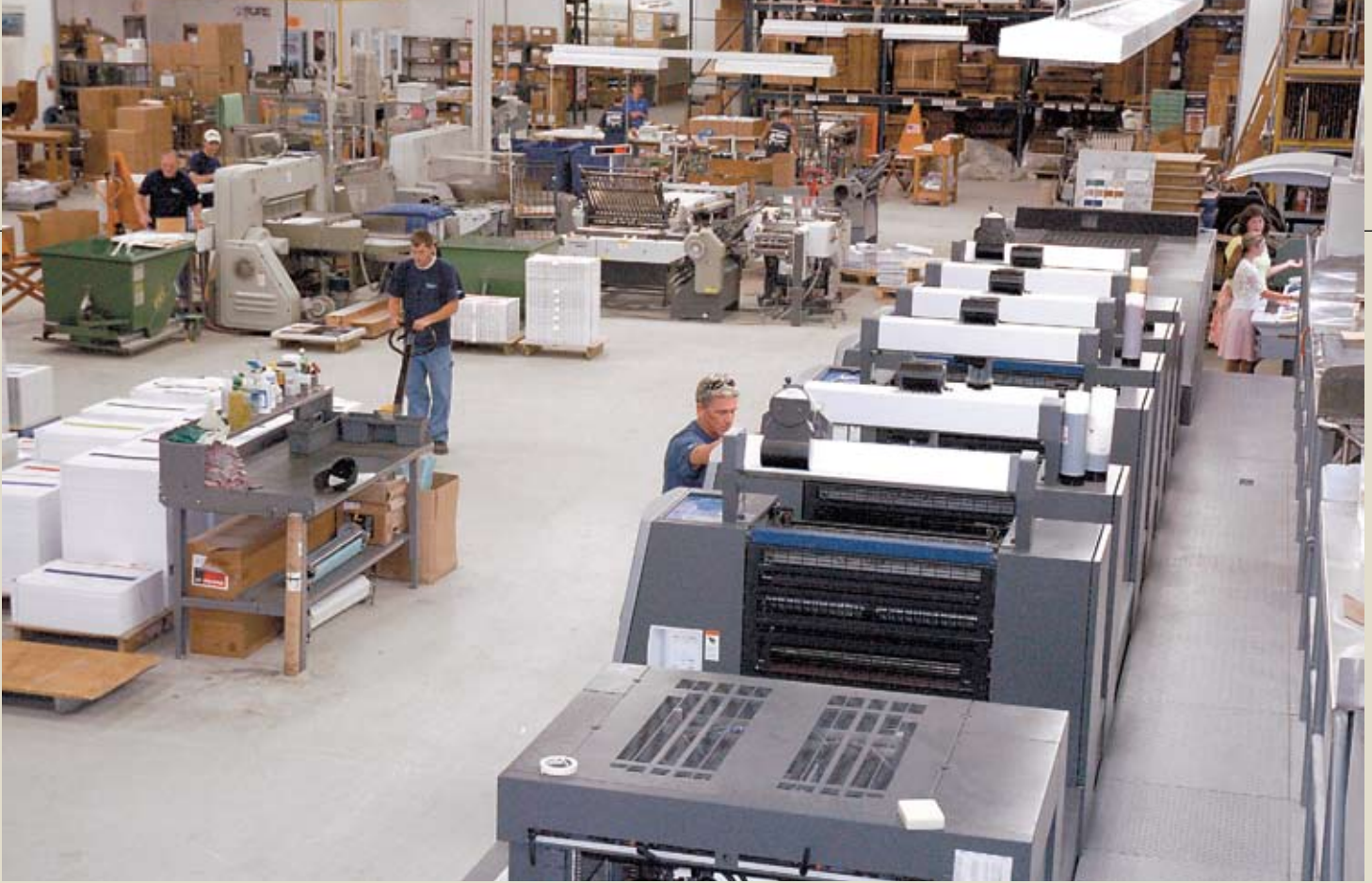
The installation of a Heidelberg Speedmaster CD74 with perfecting and in-line aqueous coating capabilities was one of the first installations in the Southeast.
